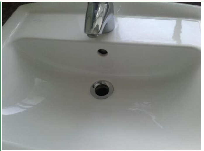
6. Bathroom, 4 bulbs not working, bath sealant mould stained, skirting chipped lhs, sink has no plug, radiator ..
