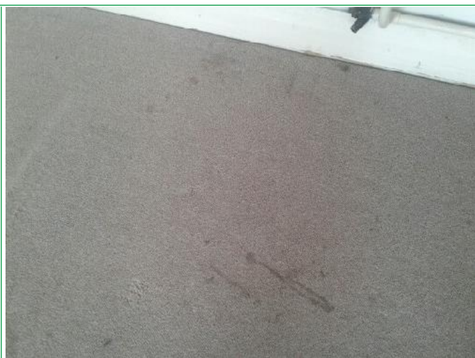
18. Bedroom, Walls patchy, finger marked around light switch, several scuffs and marks lower areas rhs, facing, ..
