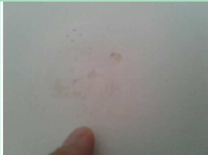
25. Lounge, Door frame chipped upper, wall finger marks around switch, some scuffs and marks lower by sockets, ..
