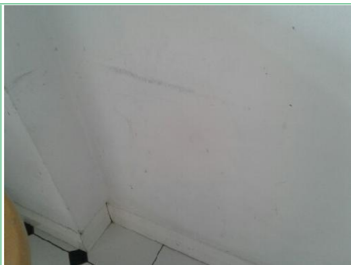
30. Kitchen, Wall spot marks by microwave, several marks rhs by door way, patch under window. Worktop ..
