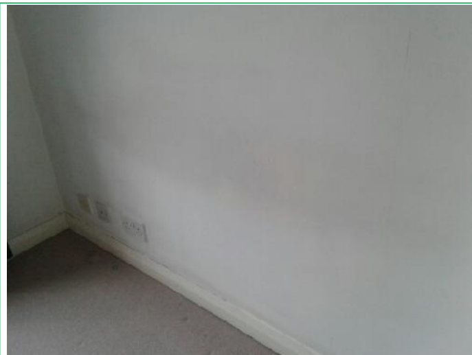
15. Bedroom, Walls patchy, finger marked around light switch, several scuffs and marks lower areas rhs, facing, ..
