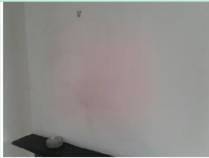
23. Lounge, Door frame chipped upper, wall finger marks around switch, some scuffs and marks lower by sockets, ..
