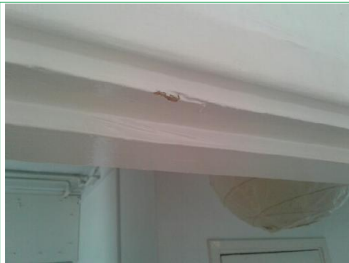
27. Lounge, Door frame chipped upper, wall finger marks around switch, some scuffs and marks lower by sockets, ..
