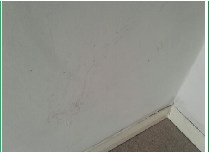
14. Bedroom, Walls patchy, finger marked around light switch, several scuffs and marks lower areas rhs, facing,..
