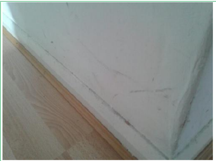
4. Hallway, Walls scuffed mid to lower area LHS, and RHS, entry phone dusty, skirting has black mark under ..
