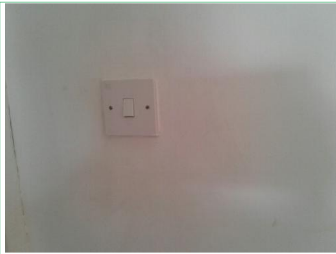
21. Lounge, Door frame chipped upper, wall finger marks around switch, some scuffs and marks lower by sockets, ..
