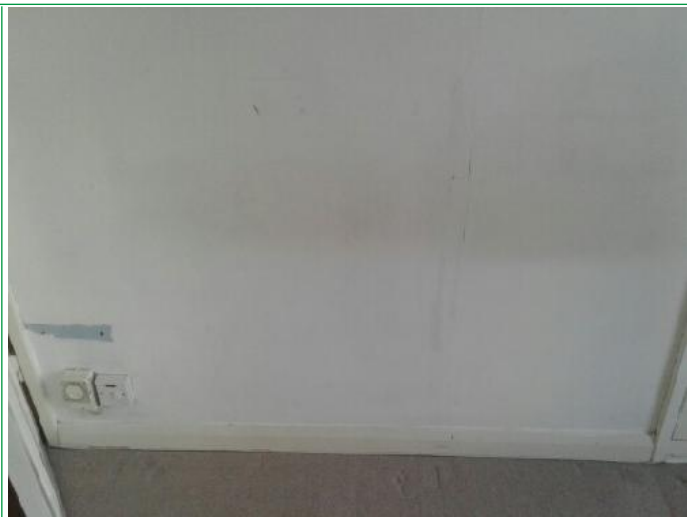
16. Bedroom, Walls patchy, finger marked around light switch, several scuffs and marks lower areas rhs, facing, ..
