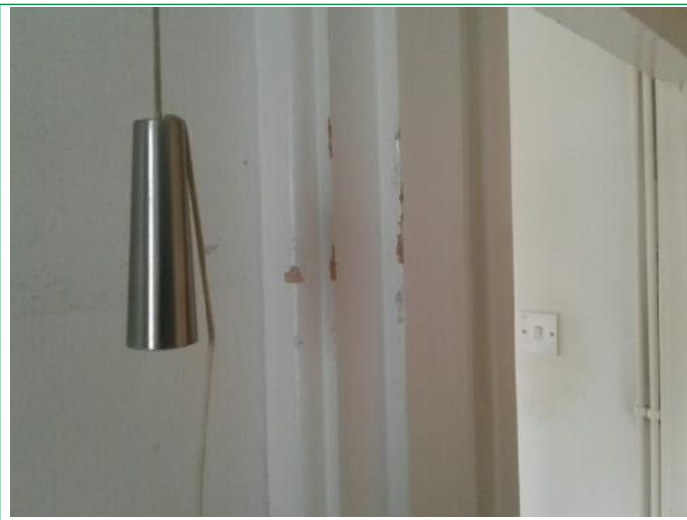
9. Bathroom, 4 bulbs not working, bath sealant mould stained, skirting chipped lhs, sink has no plug, radiator ..
