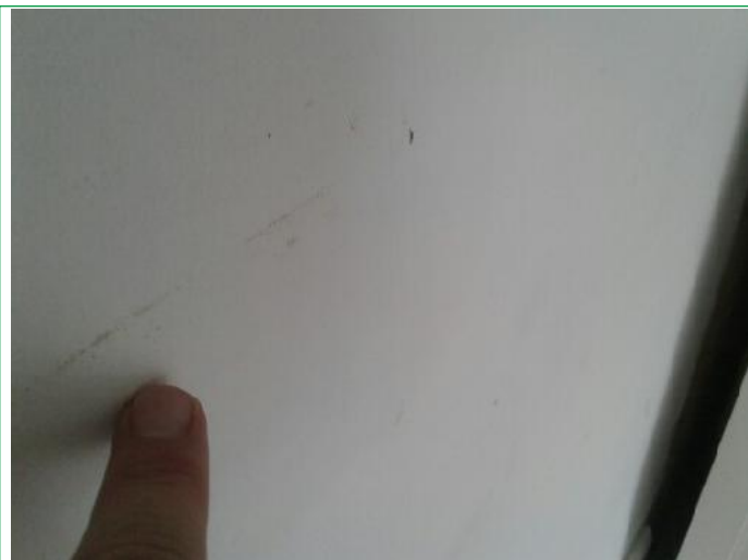
31. Kitchen, Wall spot marks by microwave, several marks rhs by door way, patch under window. Worktop chipped,..
