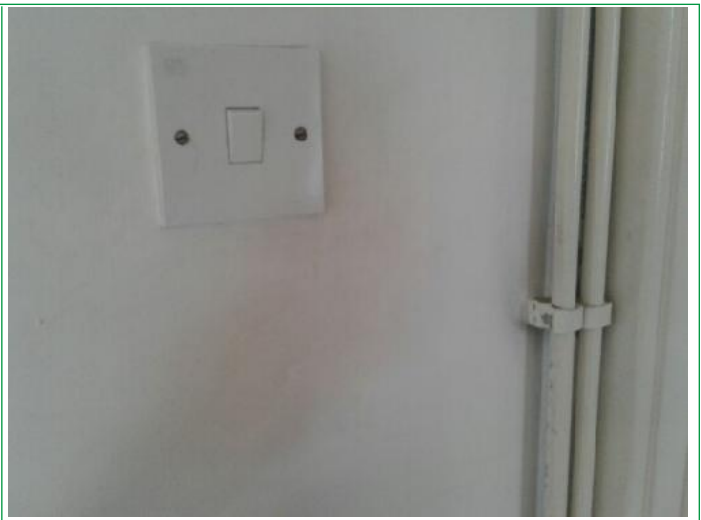
10. Bedroom, Walls patchy, finger marked around light switch, several scuffs and marks lower areas rhs, facing,..
