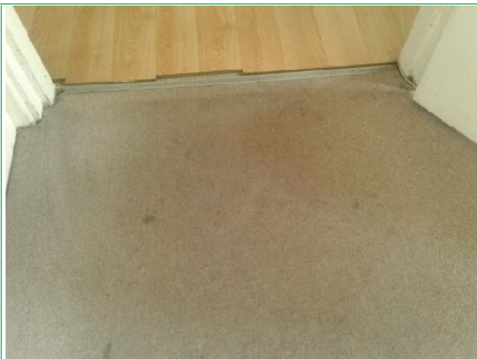
20. Bedroom, Walls patchy, finger marked around light switch, several scuffs and marks lower areas rhs, facing, ..
