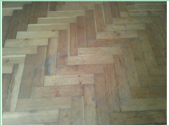
26. Lounge, Door frame chipped upper, wall finger marks around switch, some scuffs and marks lower by sockets, ..
