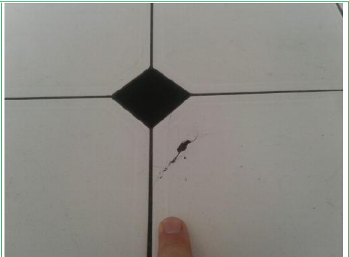
36. Kitchen, Wall spot marks by microwave, several marks rhs by door way, patch under window. Worktop ..
