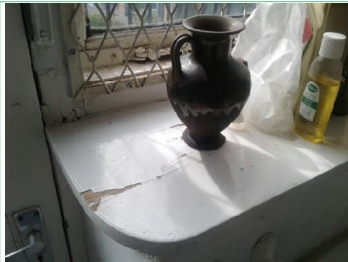
35. Kitchen, Wall spot marks by microwave, several marks rhs by door way, patch under window. Worktop chipped,..
