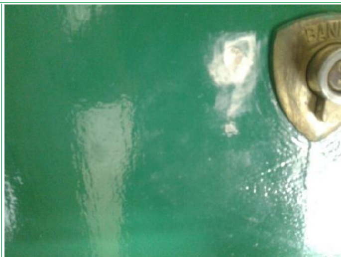
2. Hallway, Walls scuffed mid to lower area LHS, and RHS, entry phone dusty, skirting has black mark under ..
