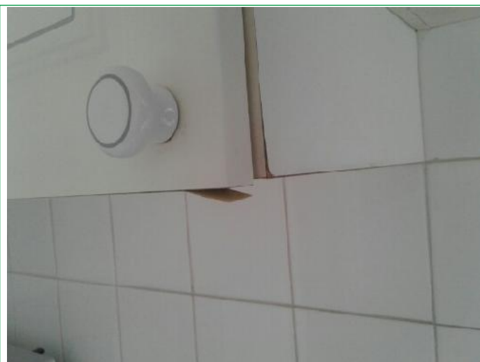
29. Kitchen, Wall spot marks by microwave, several marks rhs by door way, patch under window. Worktop chipped,..
