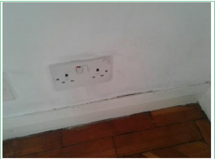
22. Lounge, Door frame chipped upper, wall finger marks around switch, some scuffs and marks lower by sockets, ..
