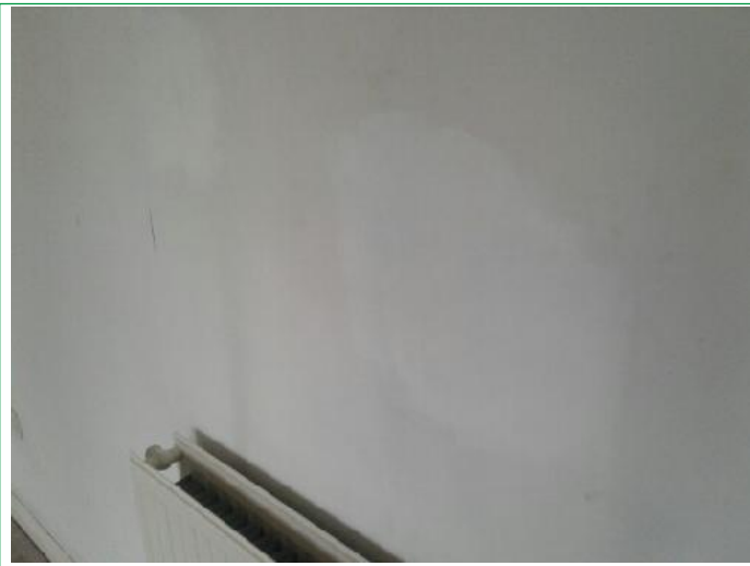
11. Bedroom, Walls patchy, finger marked around light switch, several scuffs and marks lower areas rhs, facing, ..
