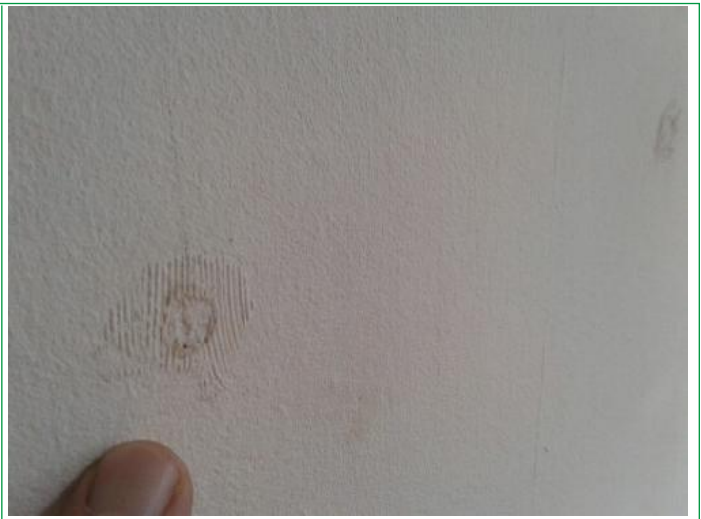
24. Lounge, Door frame chipped upper, wall finger marks around switch, some scuffs and marks lower by sockets, ..
