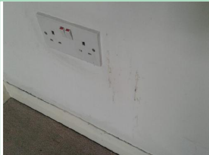
13. Bedroom, Walls patchy, finger marked around light switch, several scuffs and marks lower areas rhs, facing, ..
