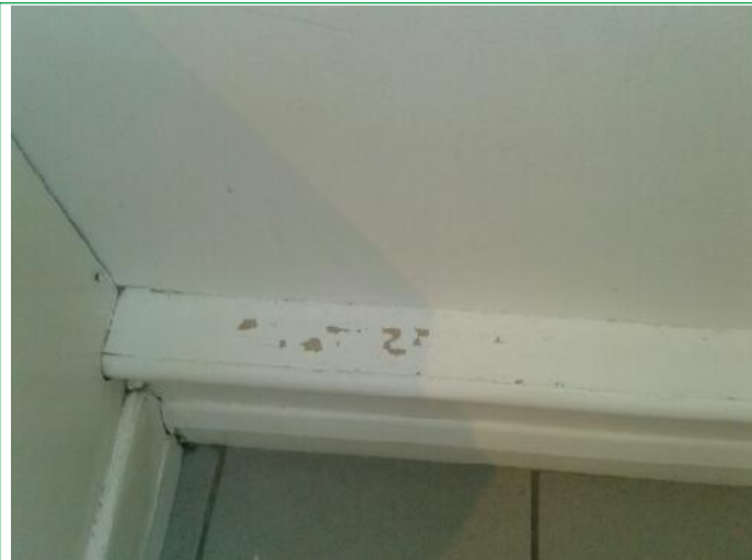
7. Bathroom, 4 bulbs not working, bath sealant mould stained, skirting chipped lhs, sink has no plug, radiator ..
