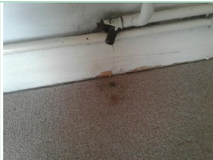
19. Bedroom, Walls patchy, finger marked around light switch, several scuffs and marks lower areas rhs, facing, ..
